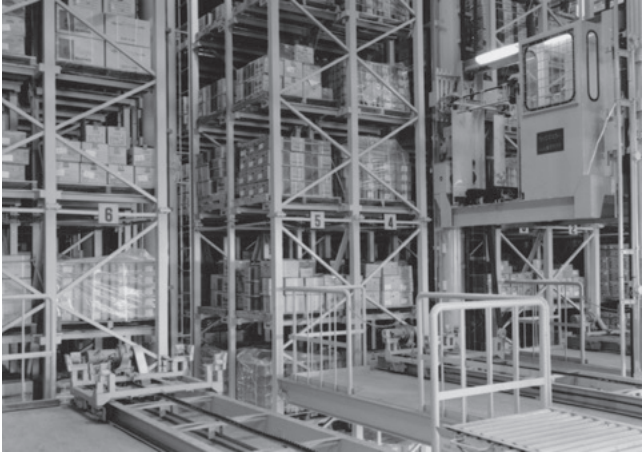
Automatic warehouse system
